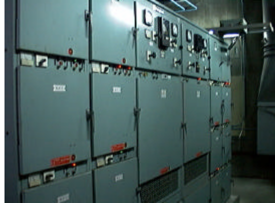
Figure 12-3 A substation inside a pier vault housing
