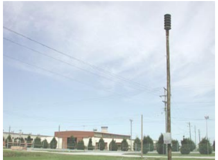
Base alert warning system.
